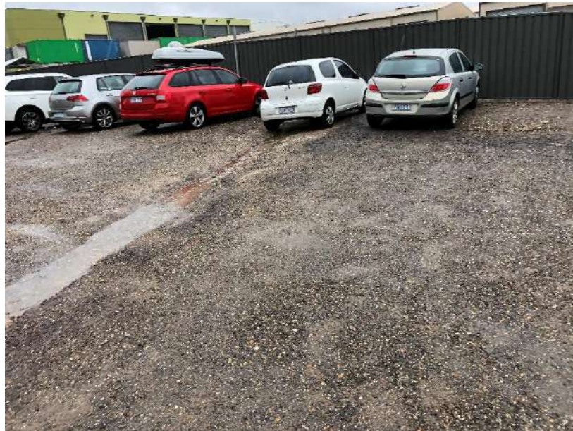
Figure 11. Depression above sewerage easement located on 14 Arnott Street, looking west. Photograph captured by Murrang Earth Sciences on 29 April 2020
